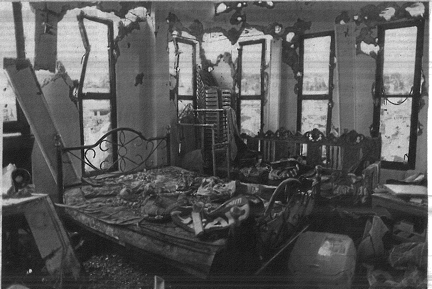
A VIEW TO A KILL Bullet-riddled bedroom of the three-story apartment where slain Abu Sayyaf leader Isnilon Hapilon reportedly stayed before all hell broke loose in Marawi City on May 23. —JEFFREY MAITEM
